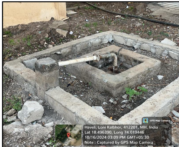
Borewell Recharge on the Campus
