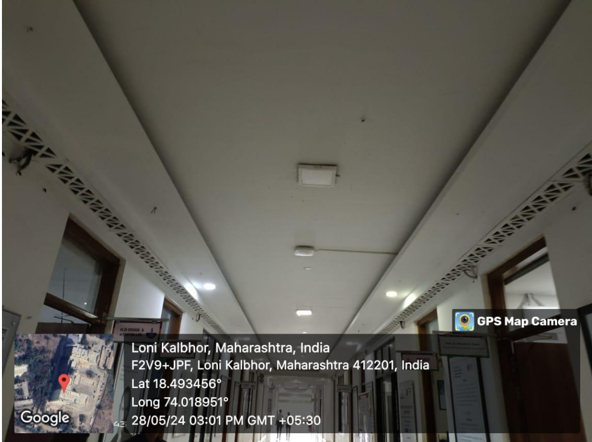
Geotagged Photograph of Sensor Based LED Bulbs
